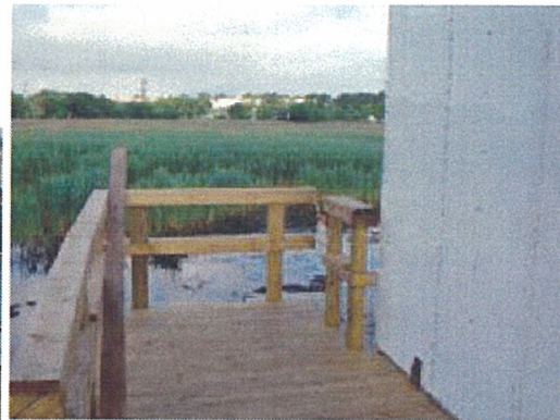
Above: Tower 2 porch looking westward. Access to the tower leg with the feed line is made from this point. An additional chain and RF hazard sign is about to be added to restrict access to this end of the porch.
