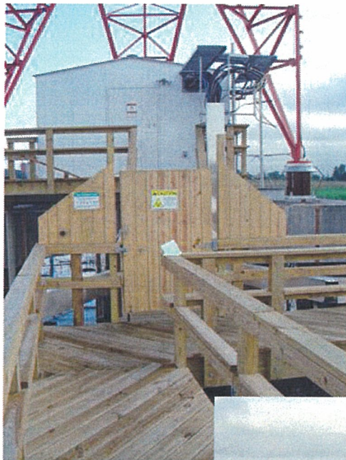
Left Center: The gate used to access Tower 2. There are stairs to the porch just beyond the gate. Each tower has a similar gate. All gates have appropriate RF safety signs. Tower 2 has the larger shelter to accommodate the phasor.
