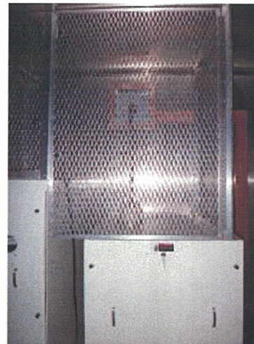
Below: All energized circuits are shielded to reduce RF field levels to a minimum and to prevent inadvertent contact.
