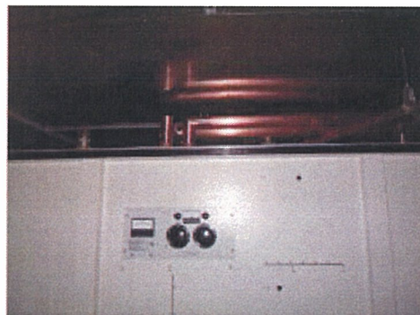
Below: The phasor cabinet, which is located in the shelter at Tower 2.
